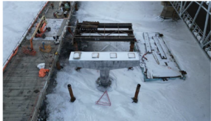
This t-shaped structure called a pier is a permanent piece of the new bridge. Three of six piers are now complete.
