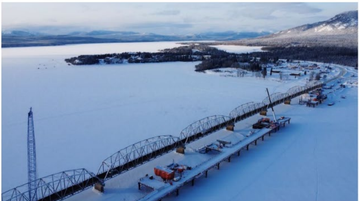
Here's an aerial view of Teslin. The wooden structure on the right is a temporary bridge used for moving equipment during construction of the new Nisutlin Bay Bridge.
